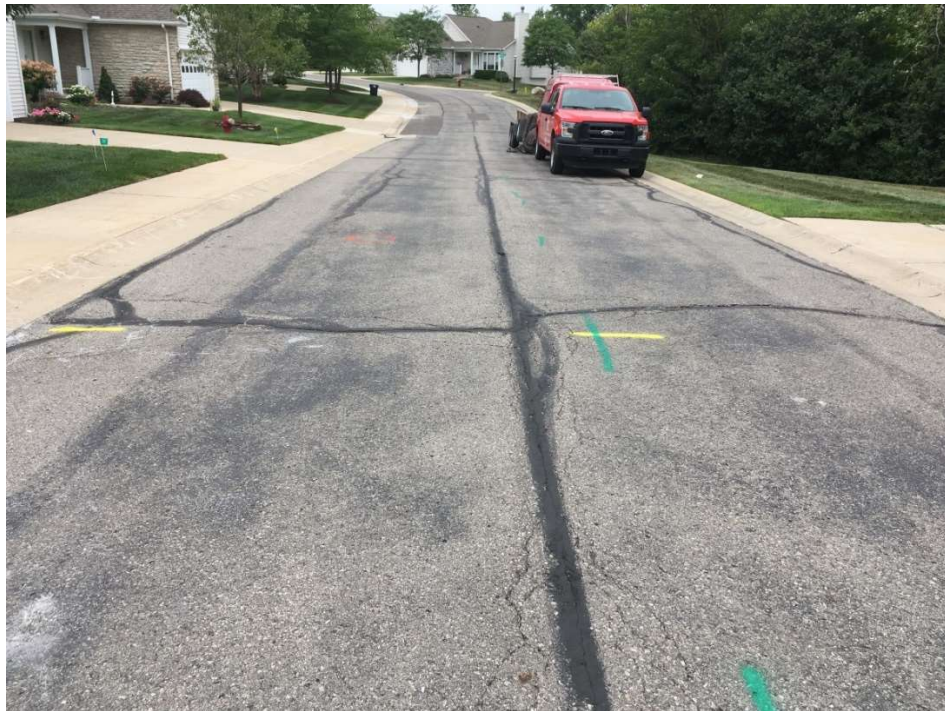
Photograph No. 8: Moderate to high severity traverse and fatigue cracking with crack sealing near boring PC-8. View to the north.
