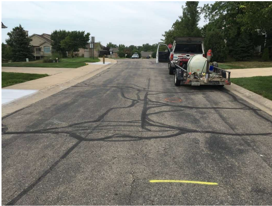
Photograph No. 5: High severity traverse and fatigue cracking with crack sealing near boring PC-5. View to the north.
