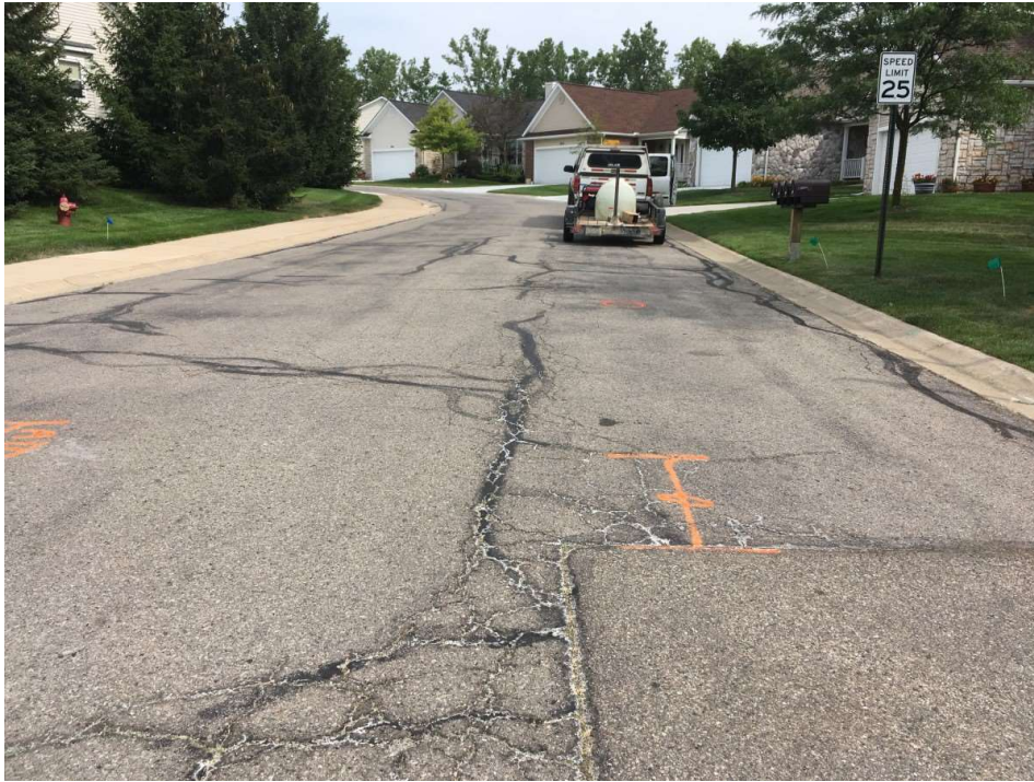
Photograph No. 1: Moderate to High severity traverse and fatigue cracking with crack sealing and areas of bituminous patching near boring PC-1. View to the north.
