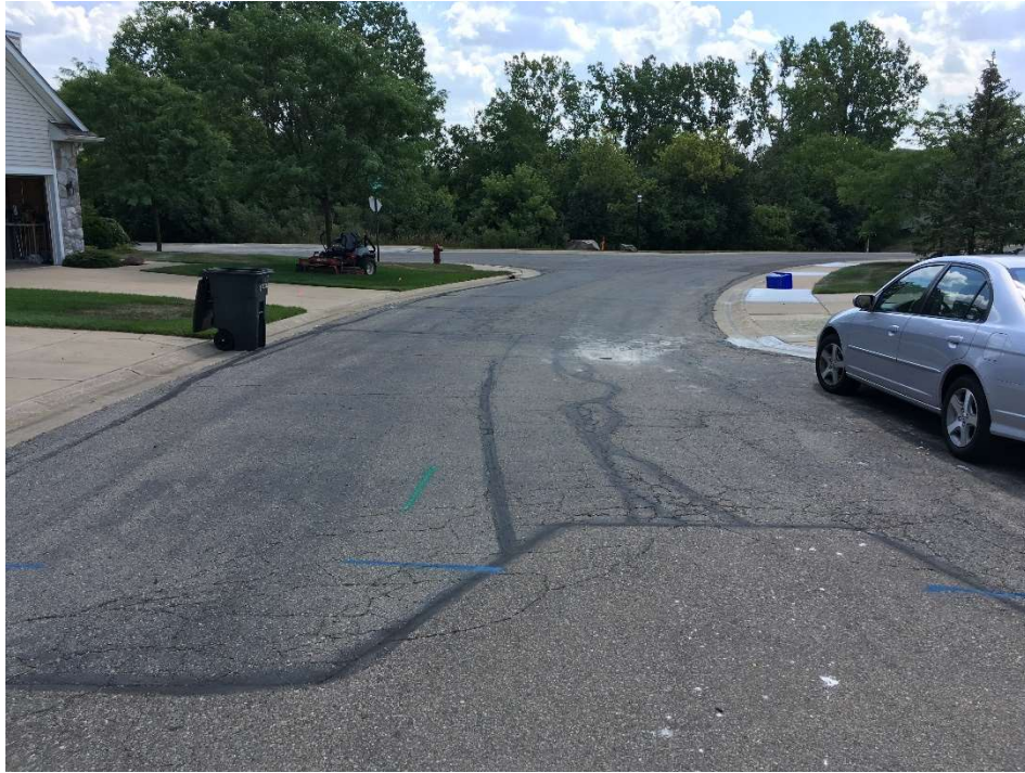
Photograph No. 7: High severity traverse and fatigue cracking with crack sealing and areas of bituminous patching near boring PC-7. View to the southeast.
