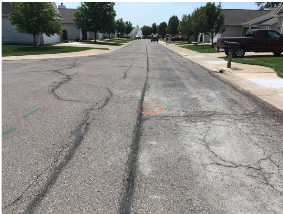
Photograph No. 4: High severity traverse and fatigue cracking with crack sealing near boring PC-4. View to the south.
