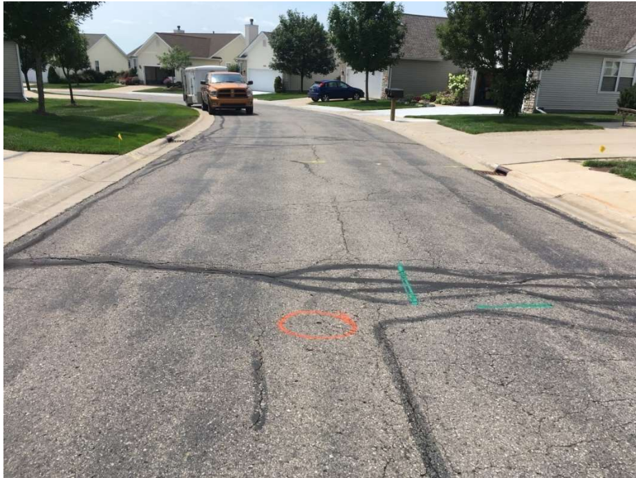
Photograph No. 3: Moderate to high severity traverse and fatigue cracking with crack sealing near boring PC-3. View to the north.
