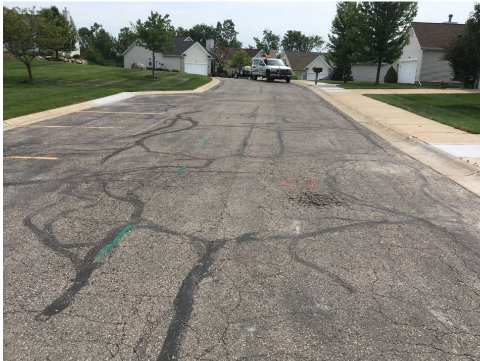
Photograph No. 2: High severity traverse and fatigue cracking with crack sealing And potholes near boring PC-2. View to the east.
