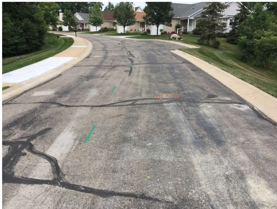
Photograph No. 6: Moderate to high severity traverse and fatigue cracking with crack sealing near boring PC-6. View to the northeast.
